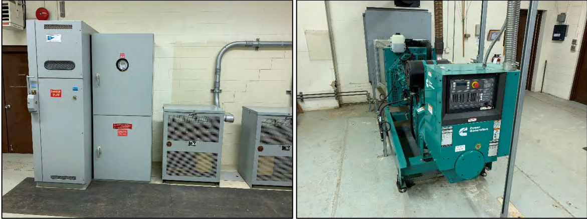
Airfield electrical infrastructure in the Field Electric Centre
