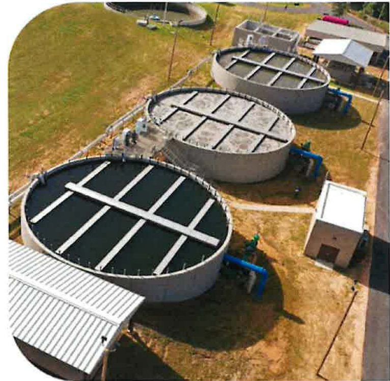
Aerial view of the AquaNereda® Aerobic Granular Sludge technology at the Wolf Creek WWTP in Foley, Alabama, in operation since January 2020
